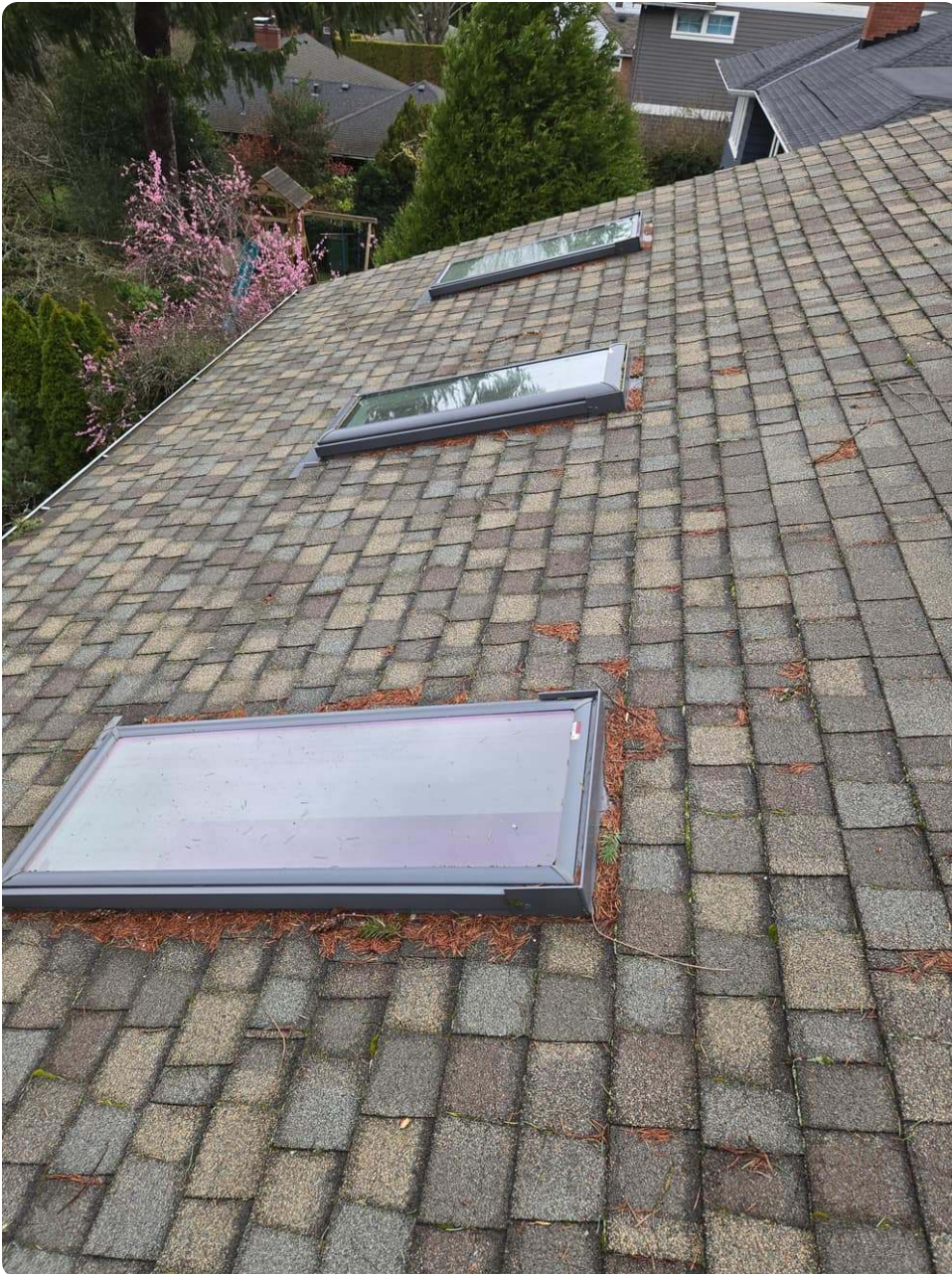
Debris building up against a skylight on an Oregon roof, a common cause of skylight leaks
