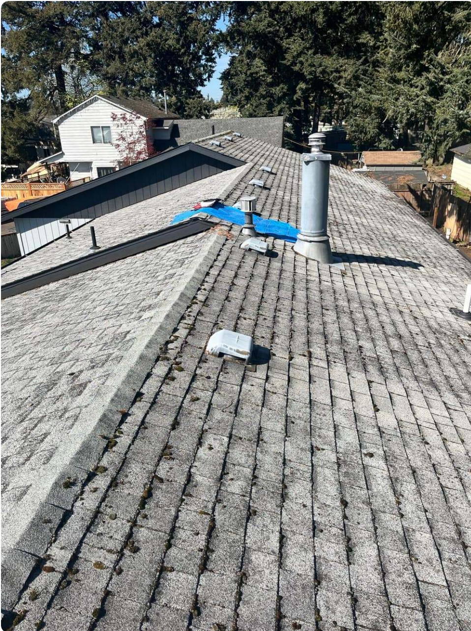
Older discolored shingles with failing flashing and an active leak, past the point of patching
