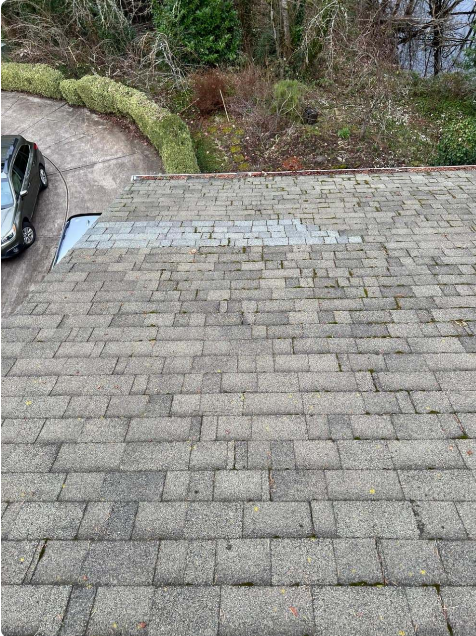
A patched section of roof, a short-term fix that's not built to last
