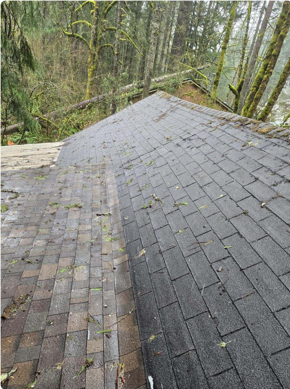
Water pooling in a shingle roof valley behind a dam of debris
