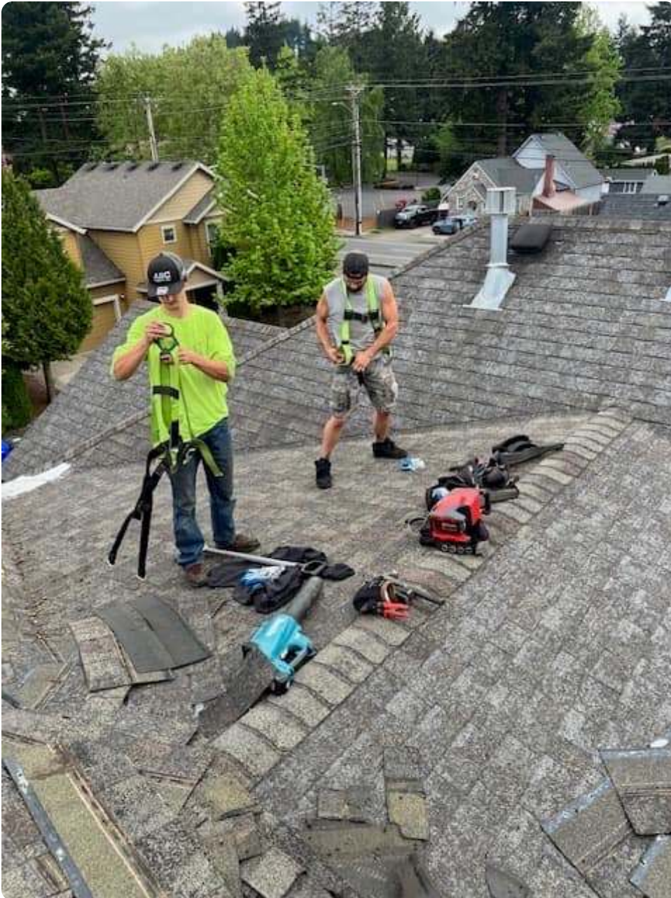
Crew members gearing up in safety harnesses before a day on the roof
