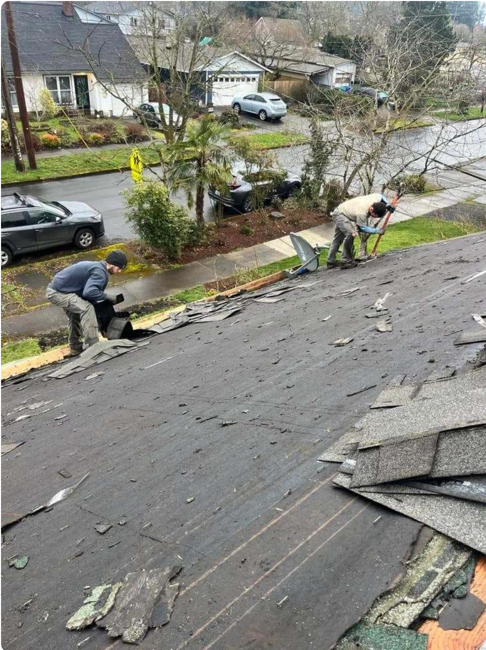
French Roofing crew tearing off an old roof down to the deck
