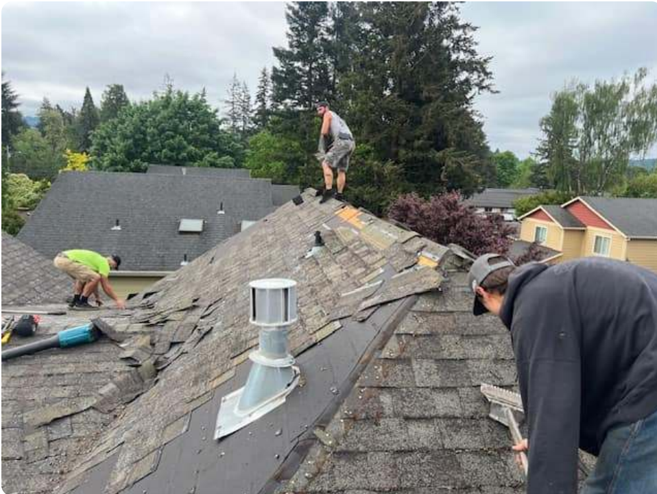
French Roofing crew mid tear-off, stripping a roof down to the deck
