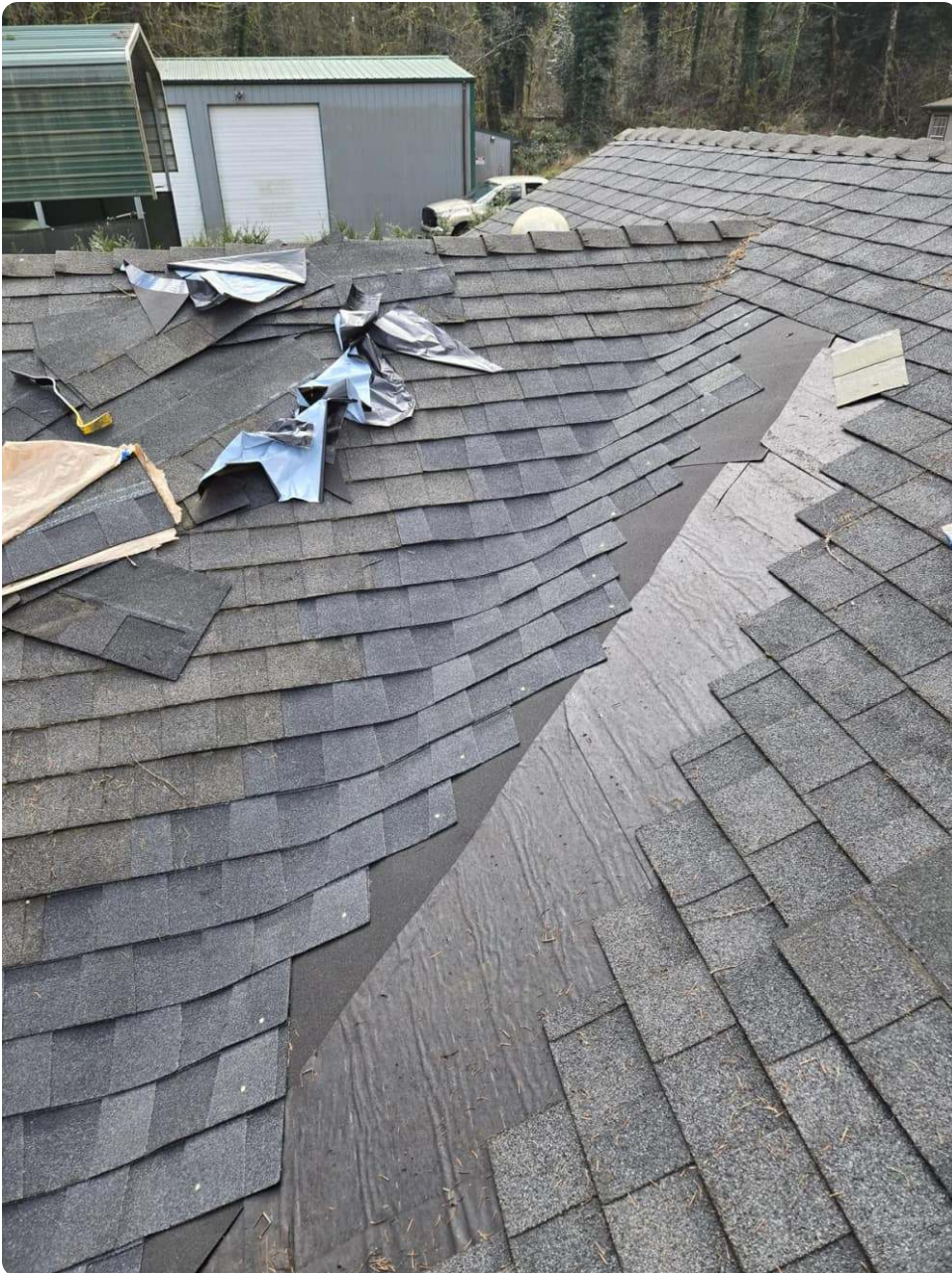
Valley installation during a roof replacement, where material and detail quality matter most
