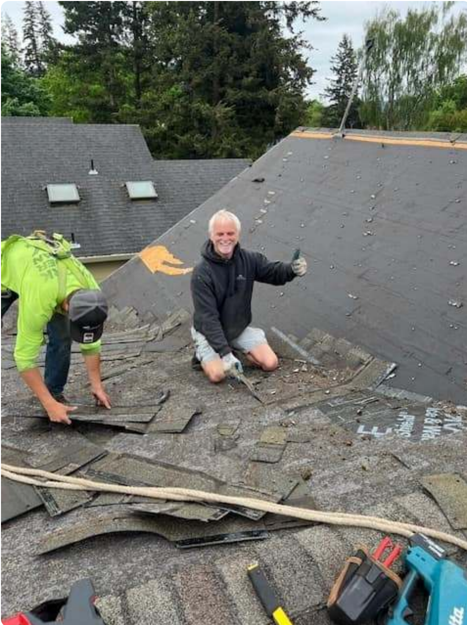
A French Roofing crew member giving a thumbs up during a roofing job
