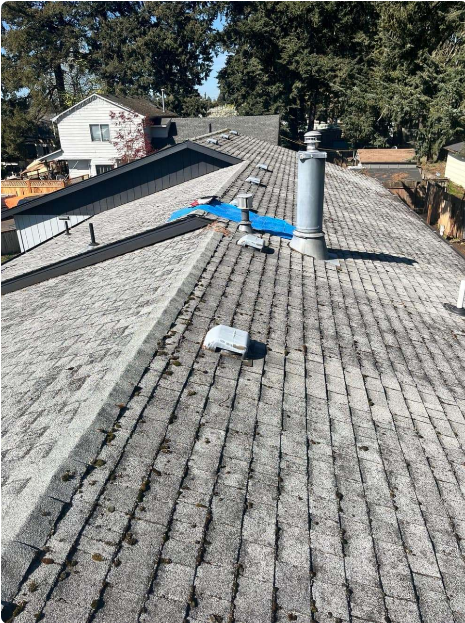
An aging roof with discolored shingles and failing flashing, past the repair-or-replace line
