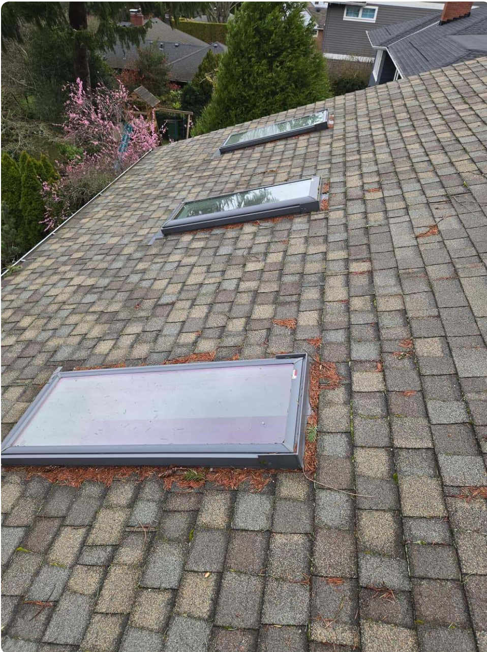
A skylight with debris collecting on its uphill side, the largest common roof penetration
