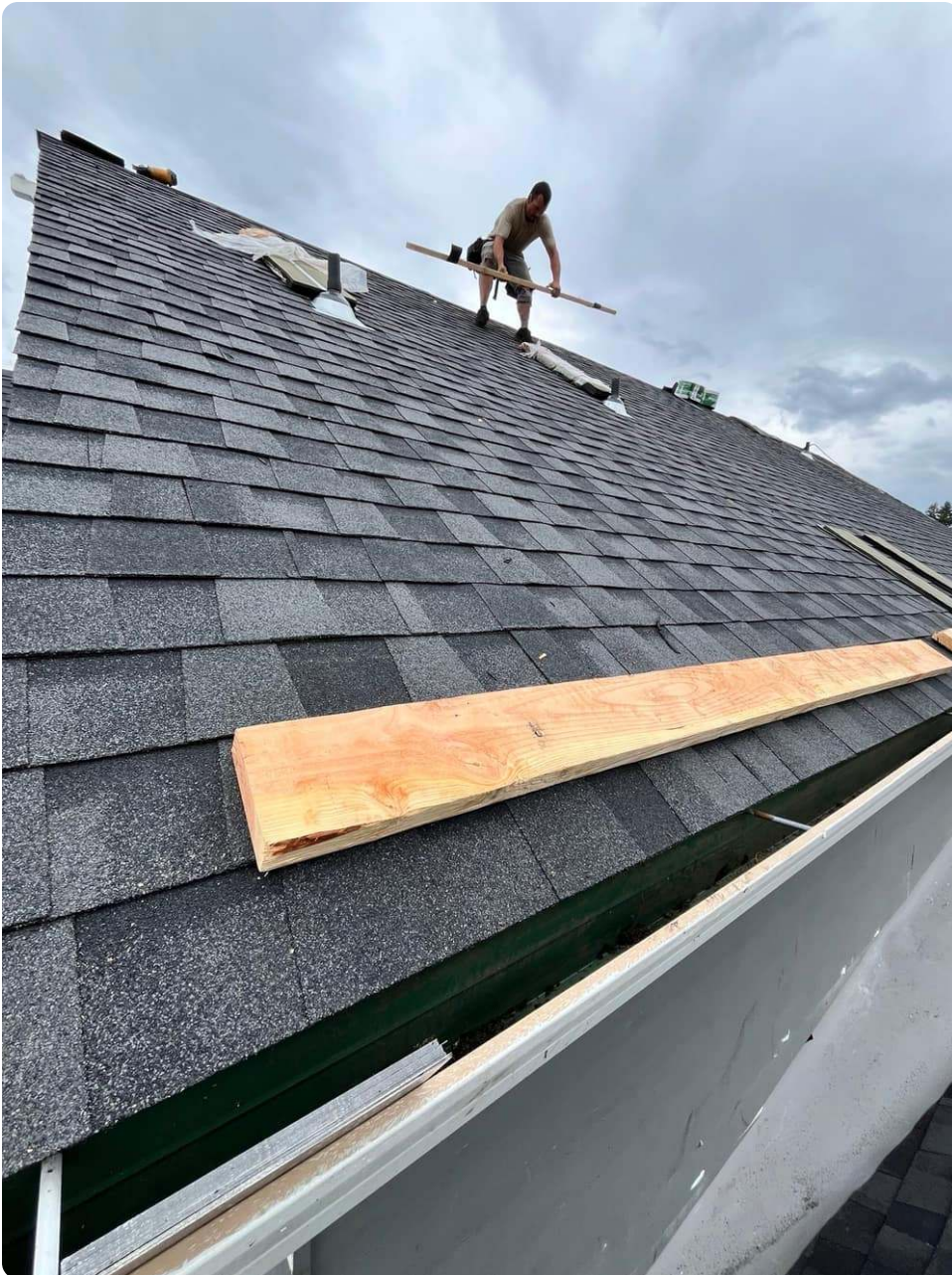
A crew member placing a new decking board during a roof repair
